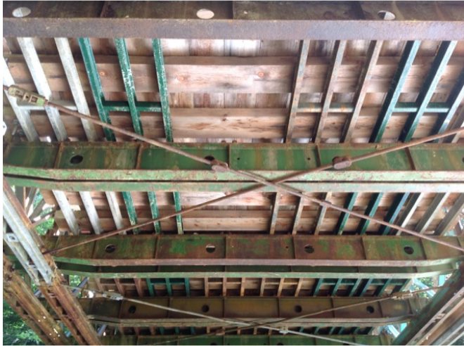
missing steel stingers
